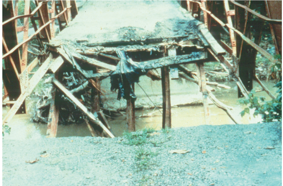
Figure P.2.21 Damaged Bridge due to Failure to Comply with Bridge Posting
